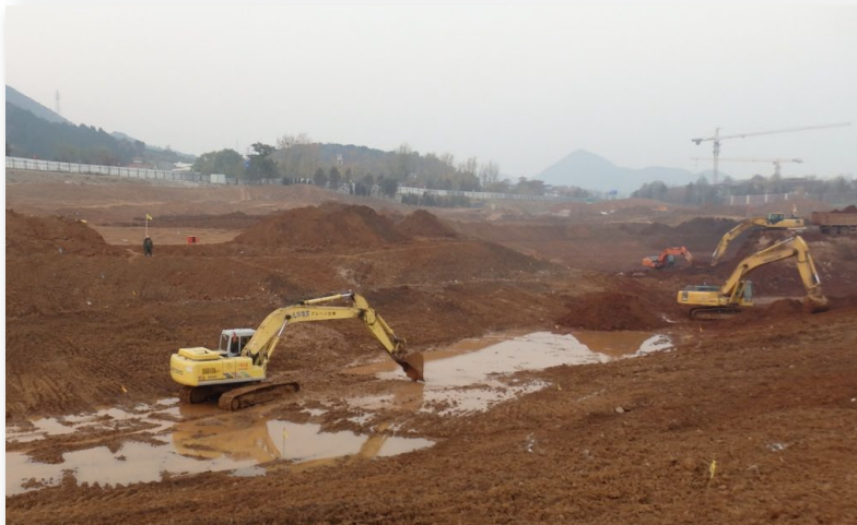
Top: Green complex construction at Longping Jiuhua Sports & Leisure Park in Changsha Middle: Team members from Flagstick and Gary Player Design go over plans with the Owner's team in Changsha Bottom: Aggressive construction at Presidential Golf Club outside of Beijing
