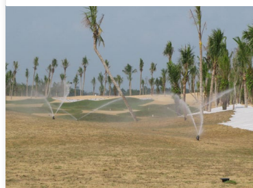
Top: Feature shaper, Dale Menning, working on the 12th green Below: Irrigation system installed and in use, with grassing underway Far left: Flagstick's Tim Zirkle and Vicky Shi after a long day onsite
