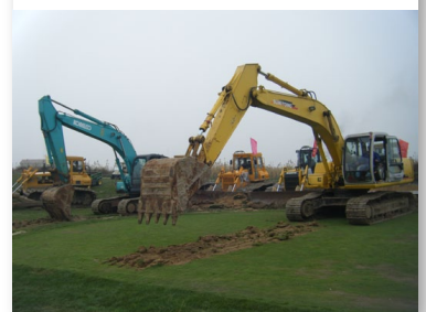
Top: Flagstick's president, Martin Moore, greeting members of the TPB team Bottom: Excavators ripping up the old to make way for the new
